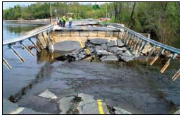
The Rainbow Lake dam was breached, resulting in an 80-ft-long collapse of the entire roadway embankment.
